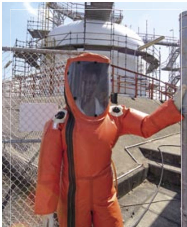
Andile Mtshiliba, in personal protection gear, prepares to enter a confined space to desludge a tetra ethyl lead tank prior to demolition, at Island View.
