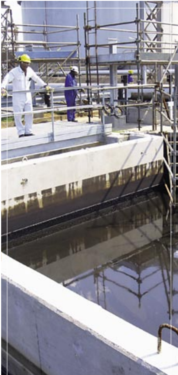
Nero Nundlal, Operations Focal Point, examines modifications to a corrugated plate interceptor (CPI) at north zone.
