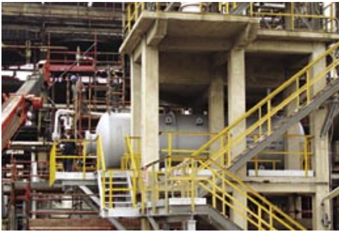
A new surge vessel was procured for the pumps on the crude distiller 2.
